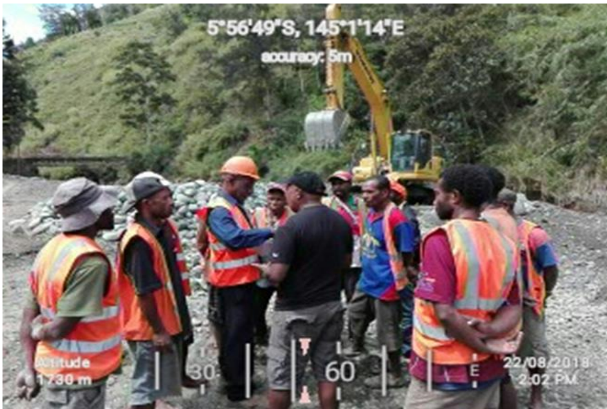
Photograph 8: A pit foreman giving instructions to local hired workers engaged in Sumbur Quarry Extraction & Crushing Site.
