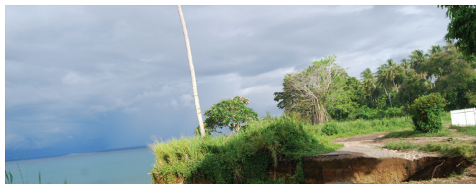
The coastal road to Pokili WMA has been eroded and the coastline has retreated many metres, threatening houses and infrastructure © Ann Peterson/Protected Area Solutions
