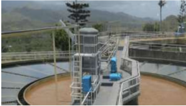
Eda Ranu's water supply treatment plant at Mt Eriama outside Port Moresby (Photo by Eda Ranu)
