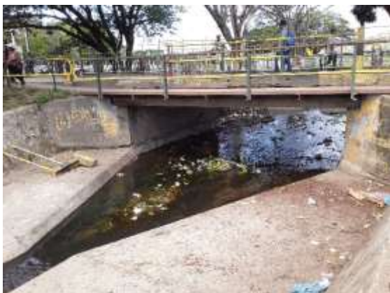
Storm water drainage in Port Moresby with growing Blue green algae
