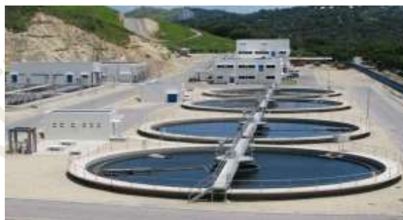
State of the art sewerage treatment plan in Port Moresby funded through the Japanese International Cooperation Agency (JICA, 2018)
