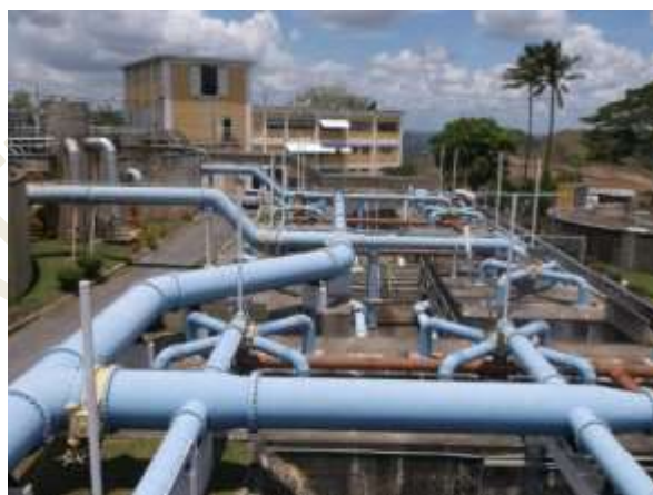
Water treatment plant operated by Eda Ranu at Mt Eriama, Port Moresby (Photo: Eda Ranu)
