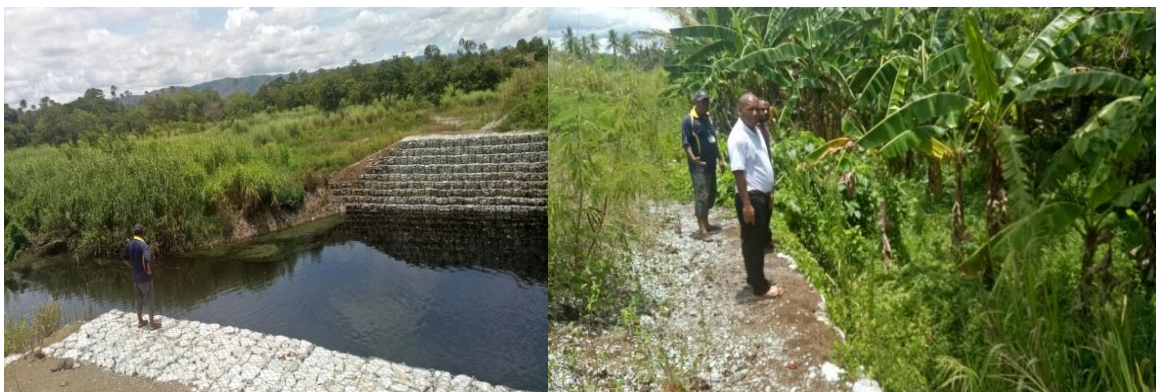
Photo 1& 2 Erosion is well protected by gabion baskets and re-vegetation on all bridge sites
