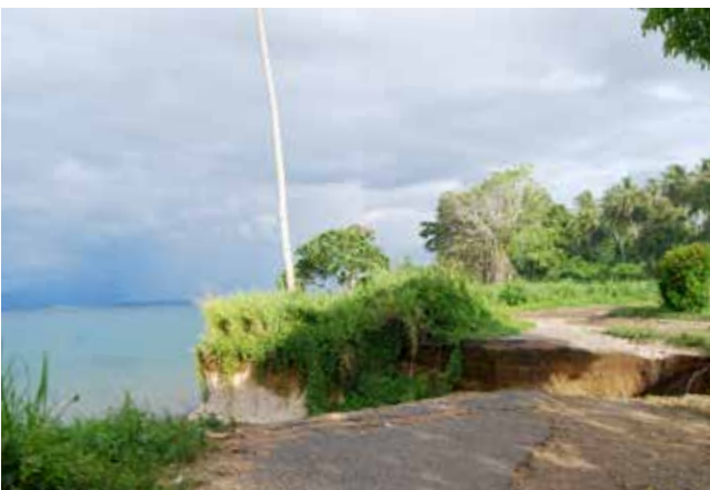
The coastal road to Pokili WMA has been eroded and the coastline has retreated many metres, threatening houses and infrastructure © Ann Peterson
