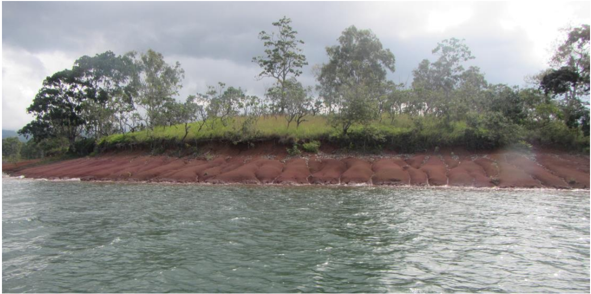
Figure 13 . Evidence of active erosion within the dam most likely due to wind wave action
