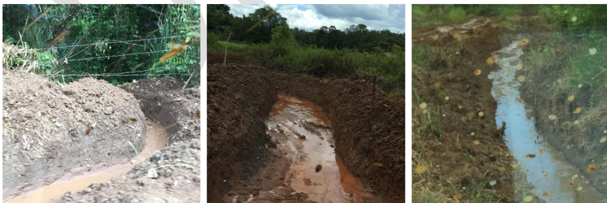
Figure 74 A sample of the multiple drains dug in order to facilitate road drainage
