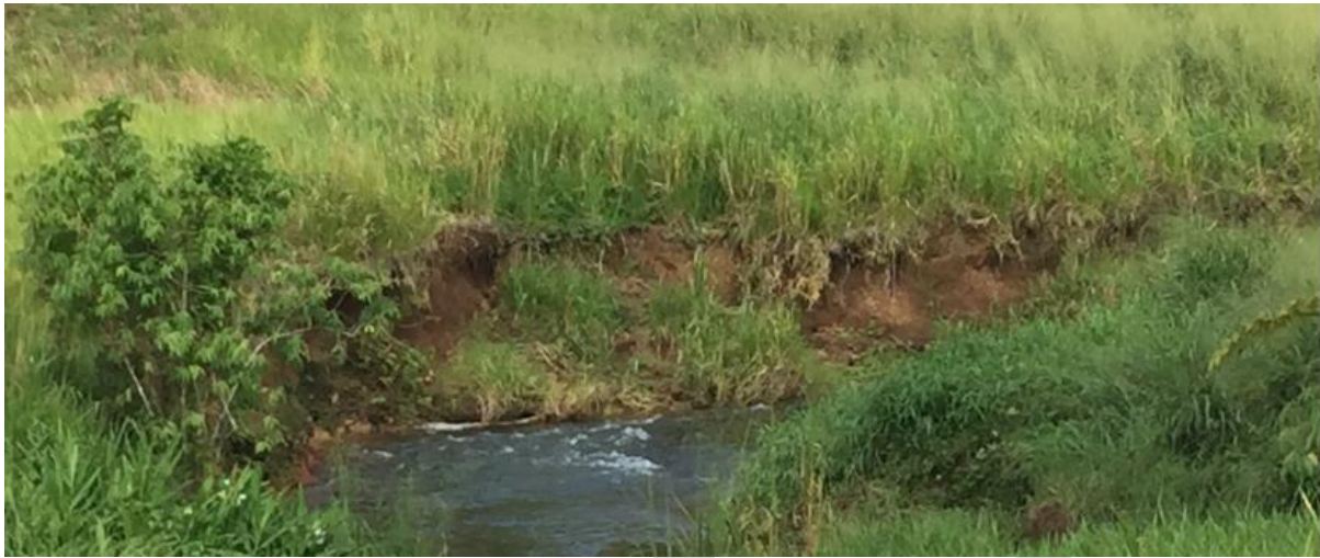
Figure 48. An example mass failure at an outer bend of Eilogo Creek, contributing to the meander development
