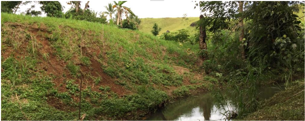
Figure 51. Staking of an eroding bank with live branches as an erosion control measure by local landholders in Sogeri.
