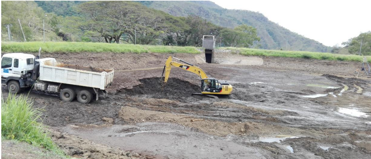
Figure 40 Removal of sediment from the first of two holding ponds along Rouna Gorge (Dec 2018).
