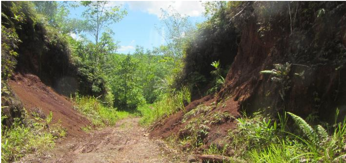
Figure 26 Multiple road cuttings along the Eilogo Creek catchment expose cohesive volcanic clays, leading to sediment slumping and transport along the road during runoff events
